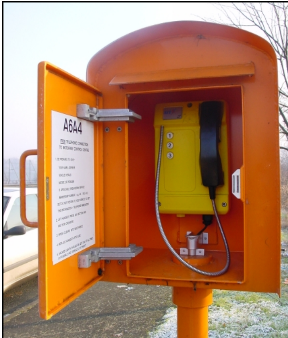
Commander telephone in BT supplied cabinet
